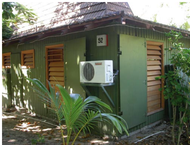
Figure 12.4 Air conditioning unit outside a tourist bungalow in Fiji *
